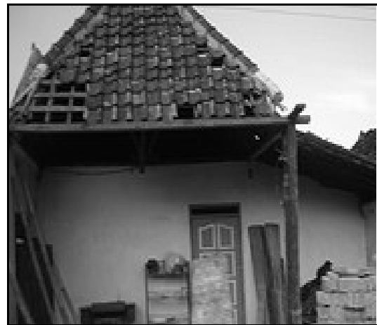
(b) Residence with tile roofing damaged due to the central Java earthquake
