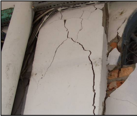
(a) Class III: crack widths of about 1.0-2.0 mm
