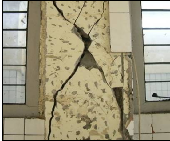
(b) Class IV: crack widths of more than 2 mm
