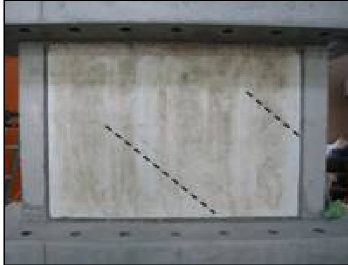
Photo 4.3. Initial damage to infilled wall.
