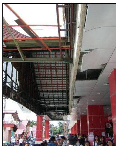
(f) Ceilings fell
