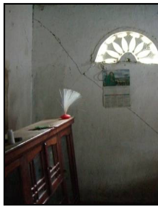
(c) Shear crack on wall
