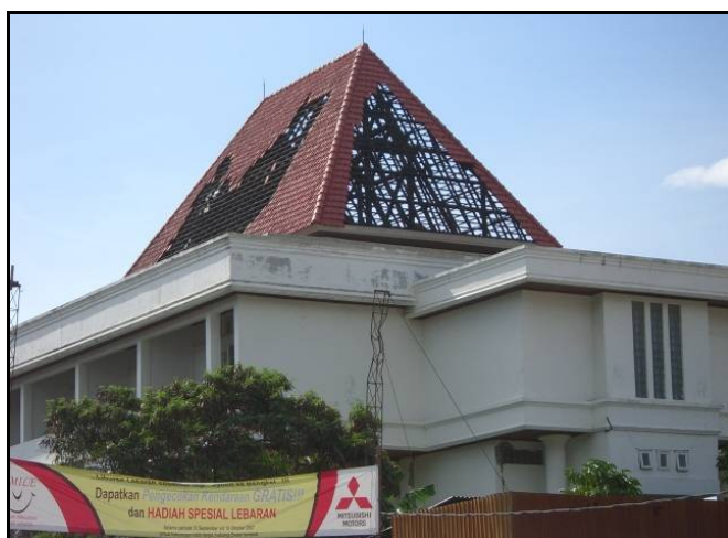
(e) Roof tiles fell
