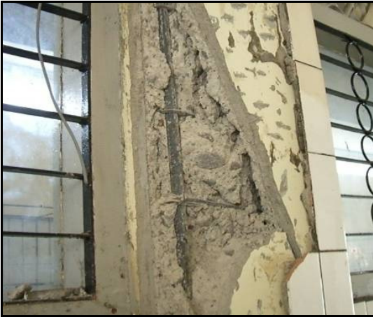
(c) Class IV: exposed reinforcing bars without buckling
