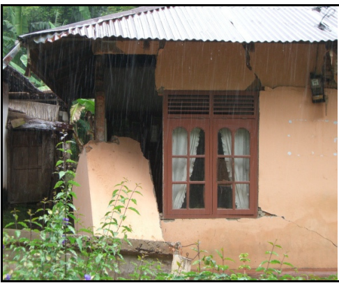
(b) Collapsed brick wall and cracks around the opening
