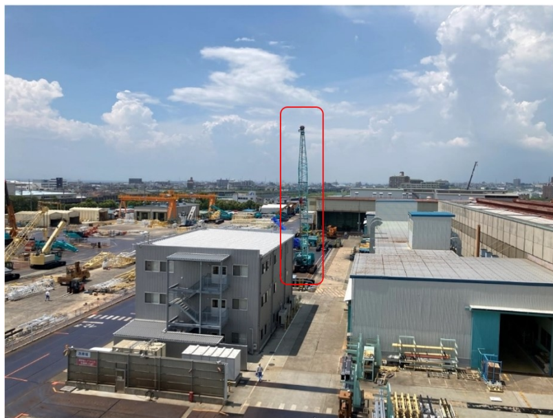
Fig. 3.34 The crane and the location where the experiment was conducted is shown.
