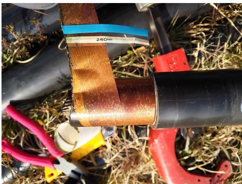
Fig. 3.11 Single core 6.6 kV crosslinked (XLPE) cable.
